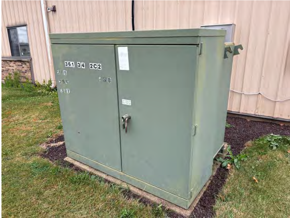
Photo 21 - View of the pad-mounted electrical transformer.
