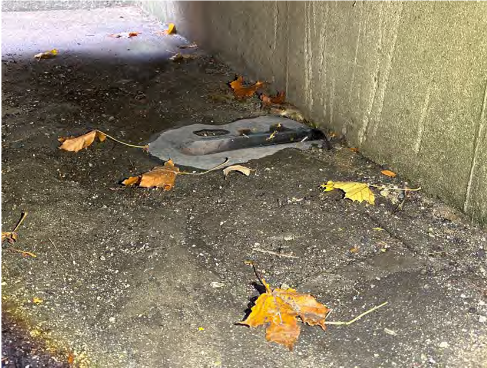
Photo 23 - View of the floor drain at the base of the exterior declining loading dock.
