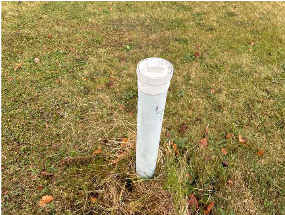
Photo 22 - View of a sewer cleanout that is located to the north of the building.
