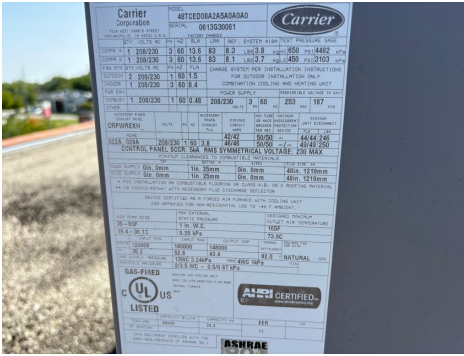
Suite 303 RTU Data Plate (2013 Carrier)
