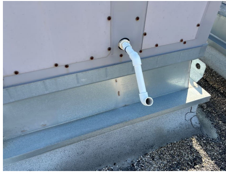
All Units Discharge to Roof
