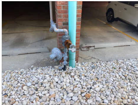
View of gas meter(s)
