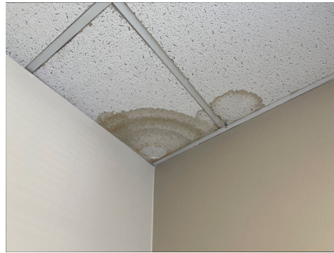
Water damage old
