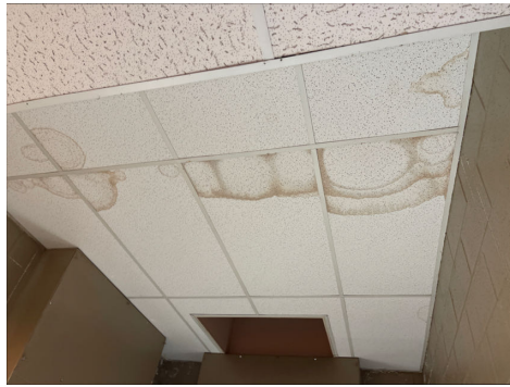
Water damage old
