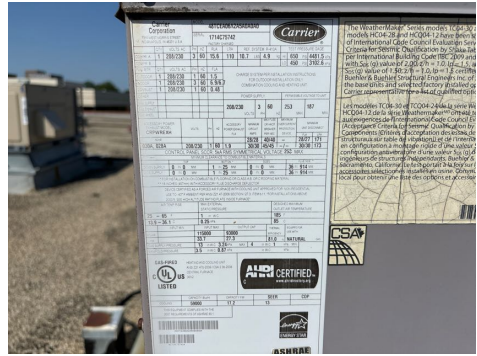
Unlabeled RTU Data Plate (2014 Carrier)
