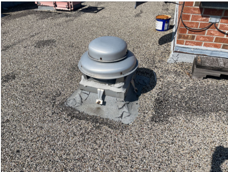
View of the ventilation
