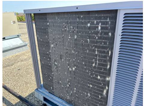
Damaged Fins-Suite 207 RTU
