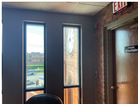
Failed Thermal Pane Seal
