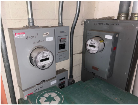
View of Electrical Meters
