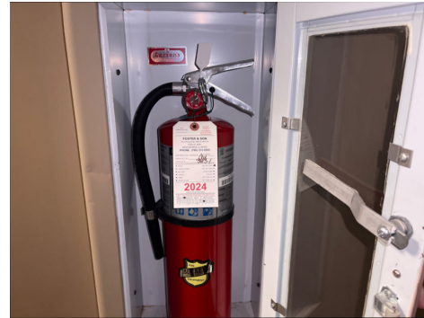
View of extinguisher
