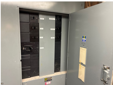
View of Disconnect Panel
