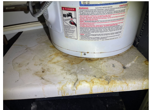
Leaking Water Heater 206
