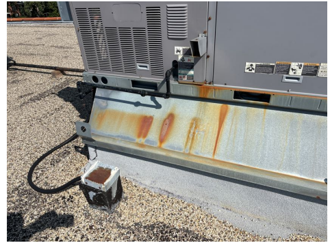
Rust/Corrosion (Multiple Units)
