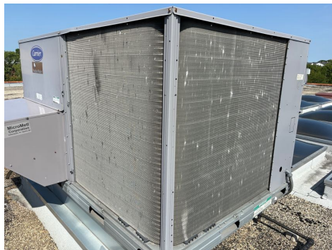
Damaged Fins-Atrium RTU
