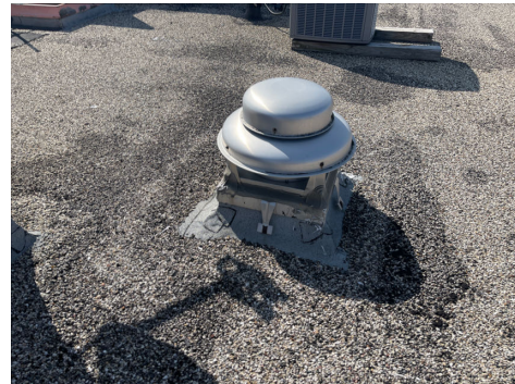
View of the ventilation
