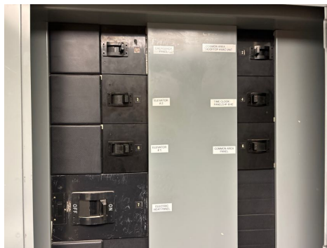
View of Disconnect Panel
