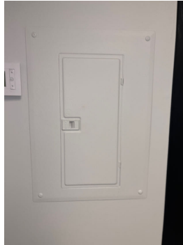
Panel 302 Painted Shut
