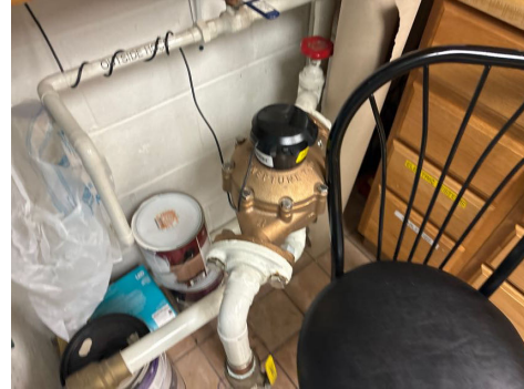
View of water Service
