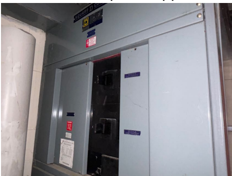
View of Service Panel
