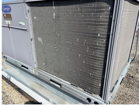
Damaged Fins-Suite 303 RTU
