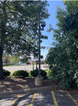
View of Lighting
