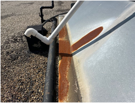
Rust/Corrosion (Multiple Units)
