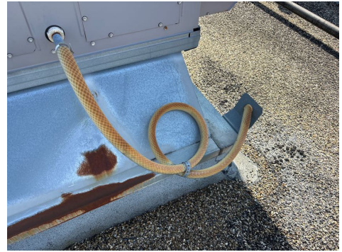
Improper Condensate Drain- Atrium RTU
