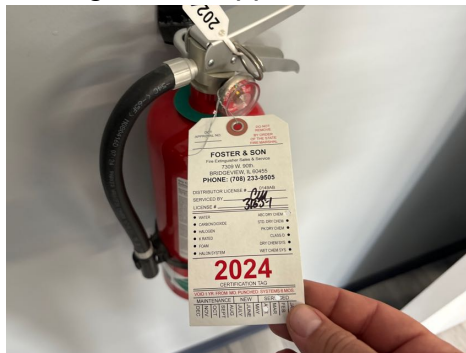
View of extinguisher
