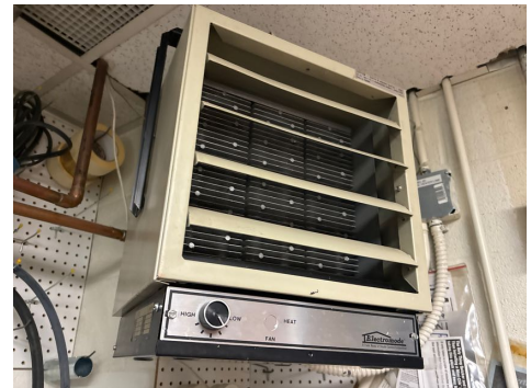
View of Mechanical Room Heater
