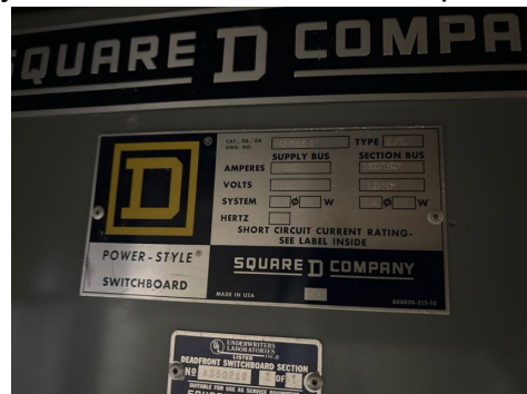
Service Panel Data Plate (800 Amp)
