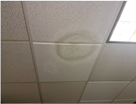
Water damage old
