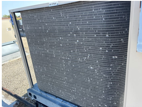
Damaged Fins-Suite 307 RTU
