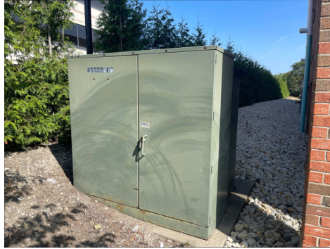
View of Transformer
