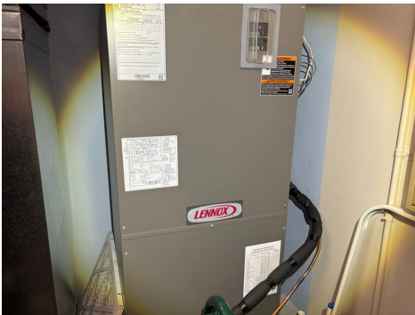
Suite 200 Air Handler
