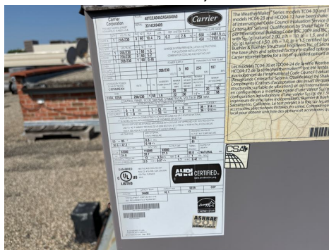
Suite 207 RTU Data Plate (2014 Carrier)
