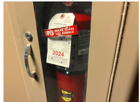
View of extinguisher
