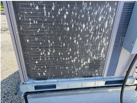
Damaged Fins-Unlabeled RTU
