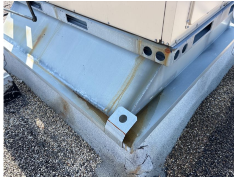
Rust/Corrosion (Multiple Units)
