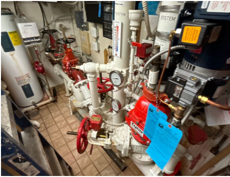
View of standpipe and sprinkler system
