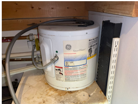
View of Water Heater
