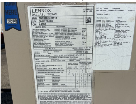
Suite 305 RTU Data Plate (2017 Lennox)
