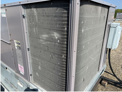
Damaged Fins-Suite 200 RTU
