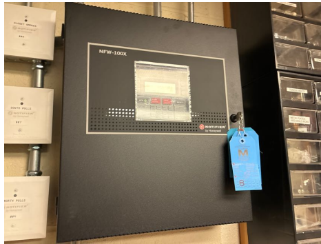
View of alarm system
