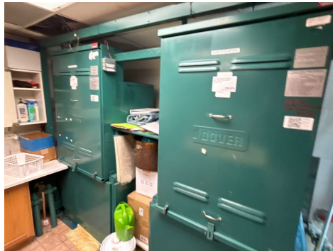
View of Elevator Motors
