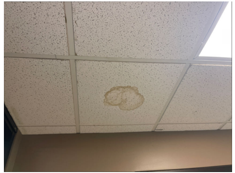
Water damage old
