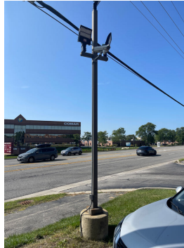
View of Lighting
