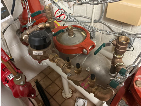
View of Water Service
