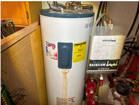
View of Common Water Heater
