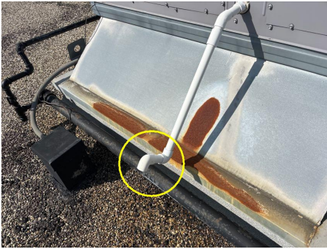
All Units Discharge to Roof
