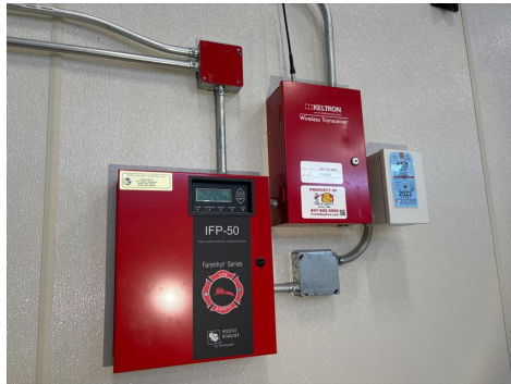
View of alarm system
