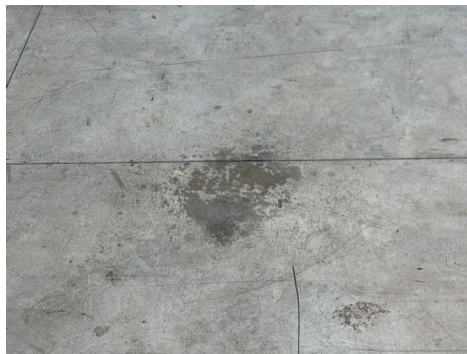
Front Infrared Heater Drip
