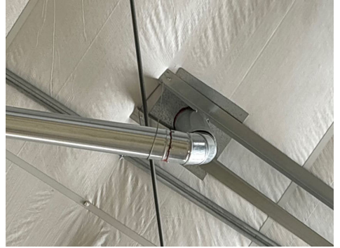
2nd Infrared Heater Drip
