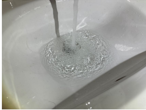
Slow Drain-Office Restroom
