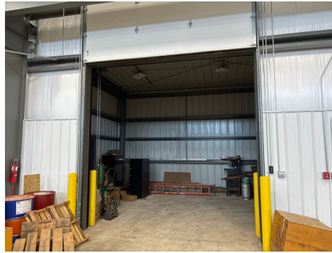
View of Overhead Doors
