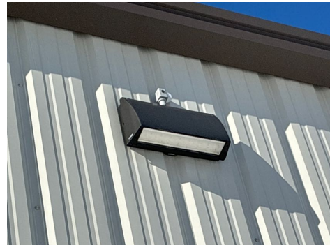
View of lighting
