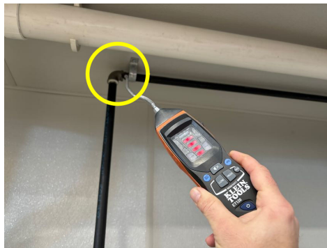
Gas Leak Noted (Near Water Heater)
