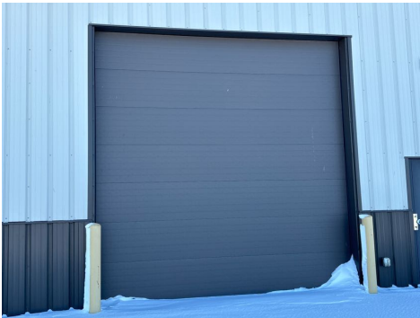
View of Overhead Doors
