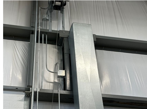
View of Ventilation Fan
