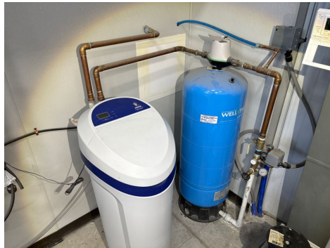
View of Water Softener
