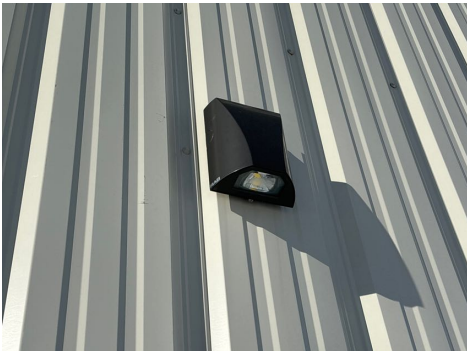
View of lighting
