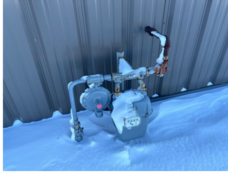
View of Gas Meter
