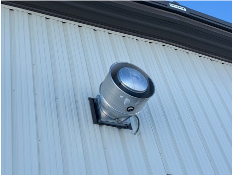
View of Ventilation Fan
