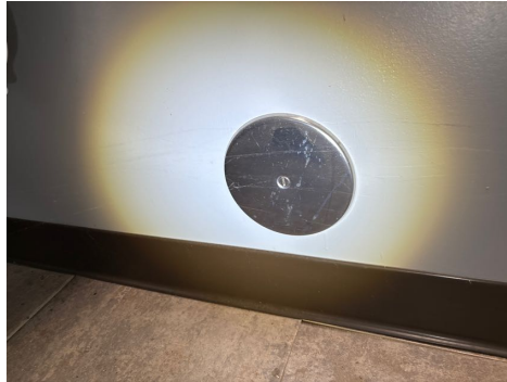
View of Possible Main Cleanout (Warehouse Restroom)
