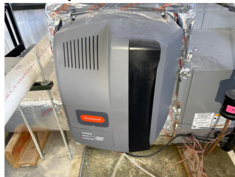
View of Humidifier
