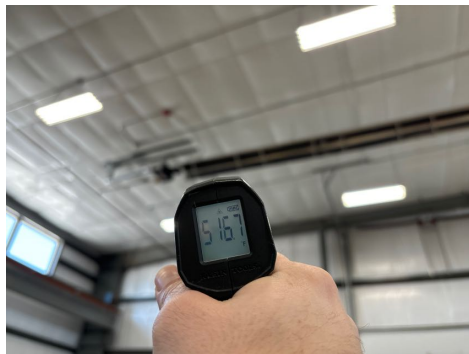
Rear Infrared Heater Supply Temp
