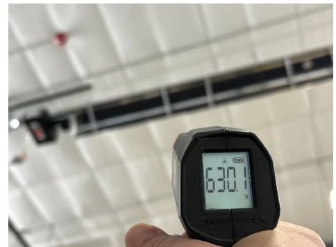
Front Infrared Heater Supply Temp
