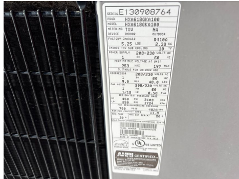
Condenser Data Plate (2013 HEIL 1.5Ton)
