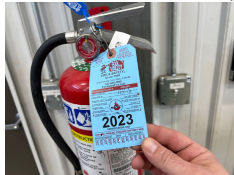
View of extinguisher
