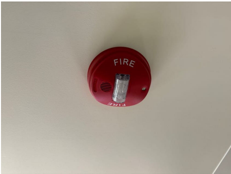
View of alarm system
