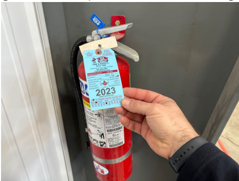
View of extinguisher
