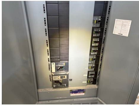
Service Panel Open
