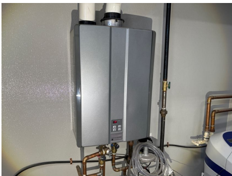
View of Water Heater
