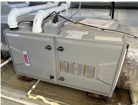
View of Furnace
