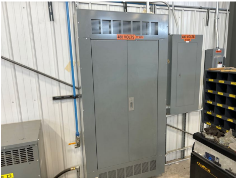
View of Service Panel
