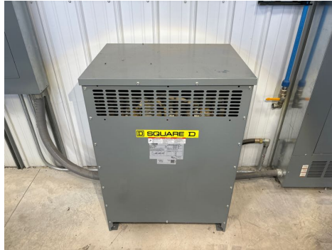
View of Transformer
