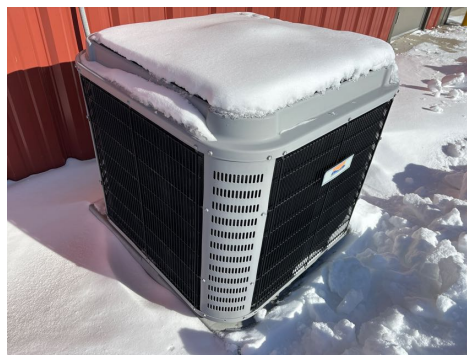
View of Condenser
