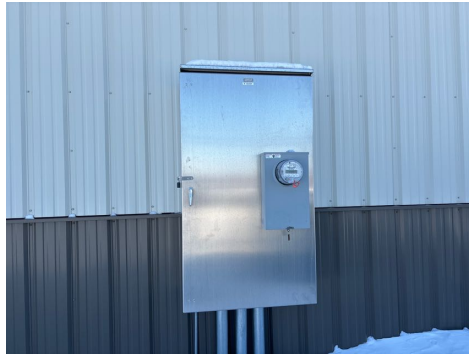
View of Electric Meter
