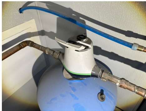
View of Water Supply
