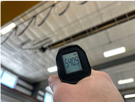
3rd Infrared Heater Supply Temp
