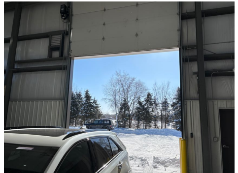
View of Overhead Doors
