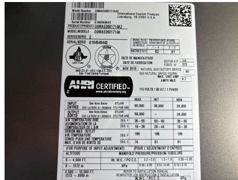
Furnace Data Plate (2016 HEIL 60k btus)
