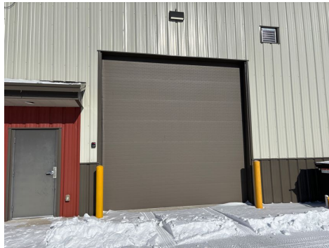
View of Overhead Doors
