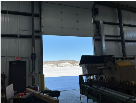
View of Overhead Doors
