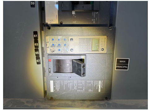
View of Main Disconnect
