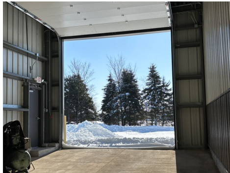
View of Overhead Doors
